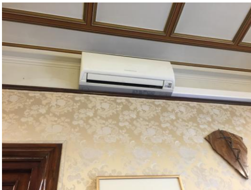
Figura 7. Unitat terminal split
