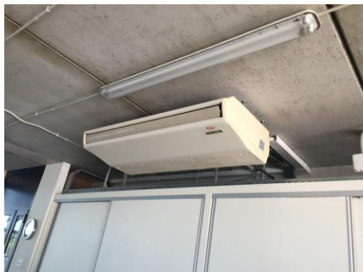
Figura 5. Unitat terminal split
